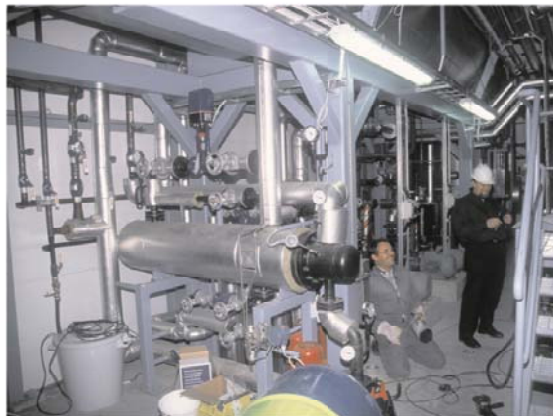
Steam station 2x 12t/h delivered to fortum riihimäki 2002
