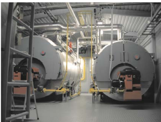
transferrable heat station 2 + 3 MW delivered to anjalankoski energia 2005
