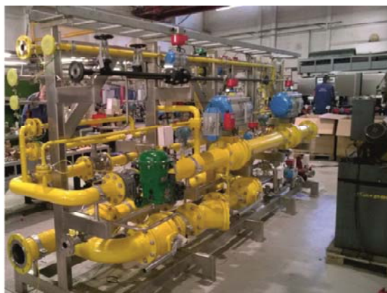
Natural gas valve station delivered to Slovakia 2014
